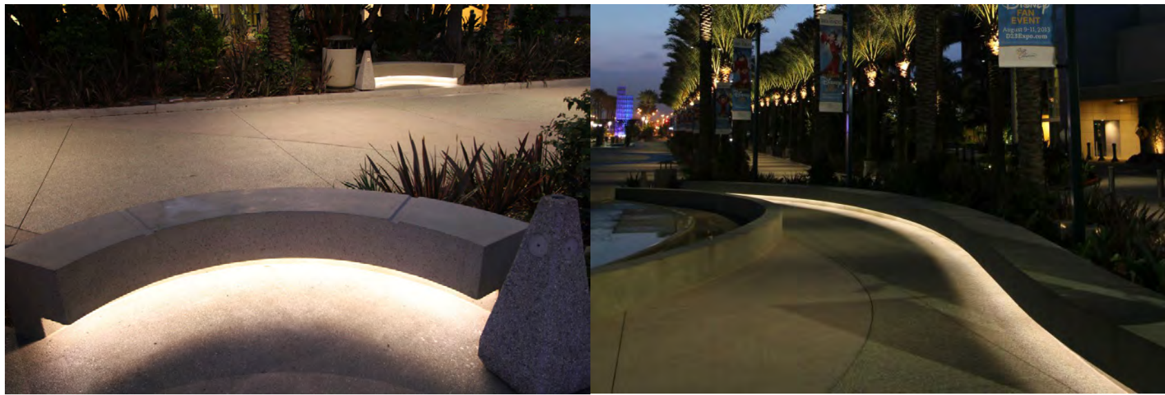
Bench Glow: Weathertight flexible LED striplighting is installed under the planter/bench toe kick area to provide a soft warm glow onto the walking surface.
